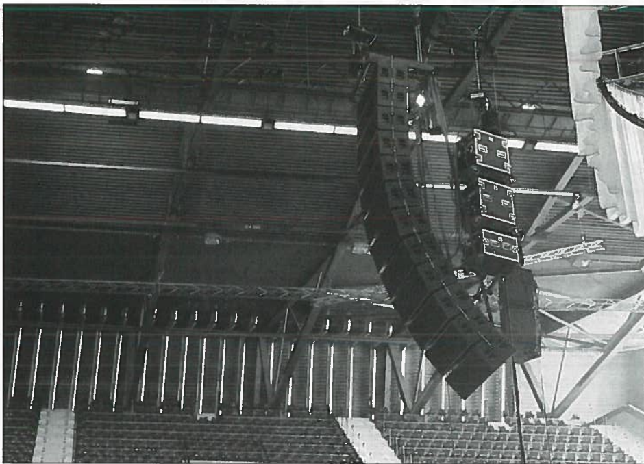
The French-built V-Dosc system flown with the amps seen clearly behind.
